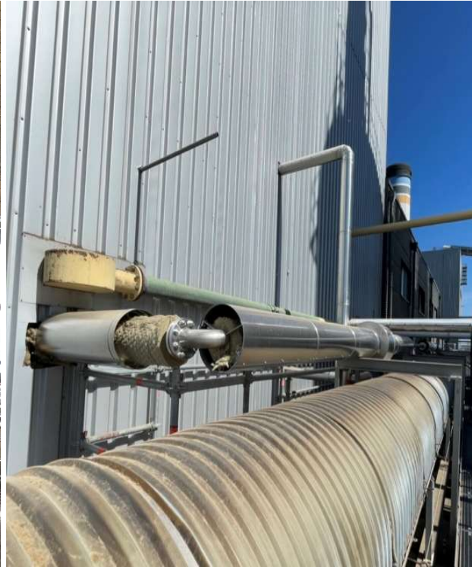
Pipe to hot-gas generator
